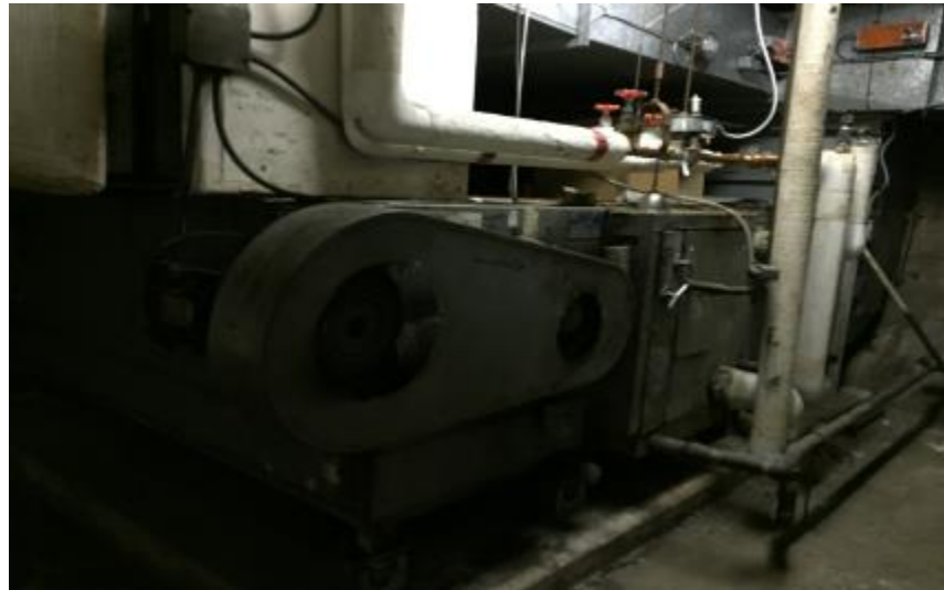
Image 5 – Air Handling Equipment
