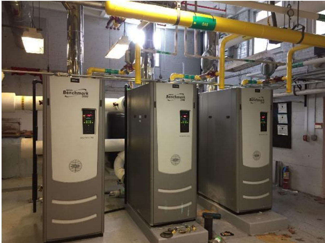
Image 3 – Hot Water Heating System
